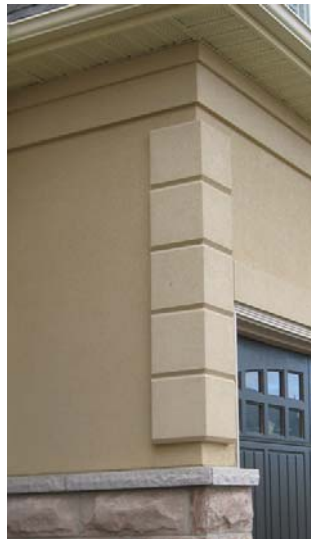
Fig. 6.3.13c - Incorrect Application of Stucco Quoining (Uneven Spacing)
