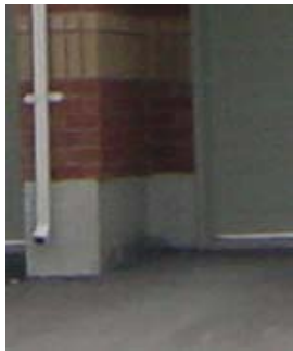
Figure 6.3.6b - Unacceptable Foundation Wall Height (at garage)
