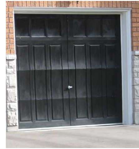
Fig. 6.3.14b - Image of Low Quality Garage Door (With Evident Warping) Not Permitted
